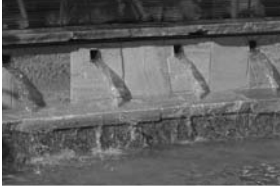
Line of plumbed PC Spillways.
